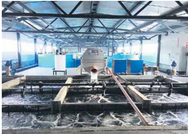
Moving bed biological reactors receive screened water directly from the drum filter.
