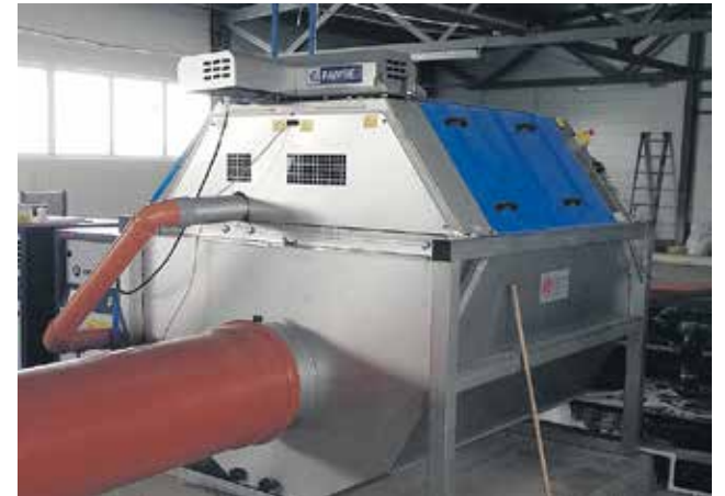
Microscreen drum filter receives water from the growout tanks.
